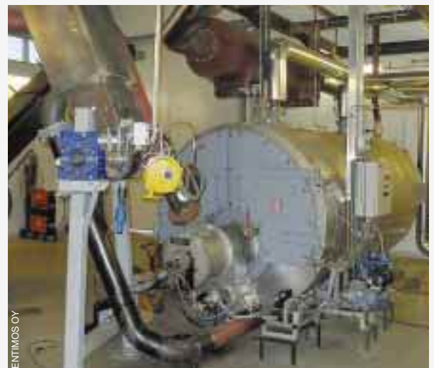
The boiler burns the gases with tar and feeds thermal kW to the municipal district heating system.
